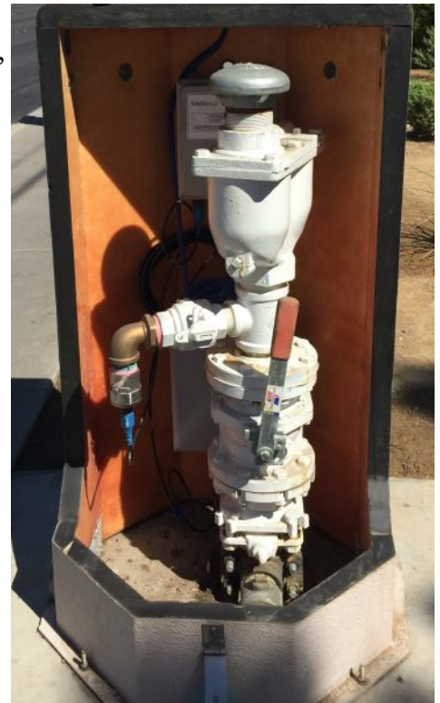
Echologics pipeline monitoring systems precisely identify and locate emerging leaks so that repairs can be made before more significant failures occur. Photo courtesy of the Las Vegas Valley Water District.
