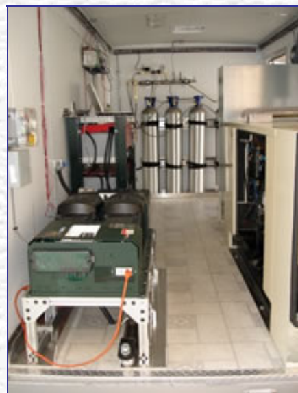
Hydrogen Off-grid System
