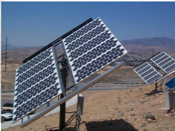
PV Arrays at Dandini Campus
