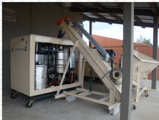
Biomax 15 Gasification Unit
