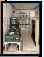
The H 2 RE system is housed within a trailer for portability.
